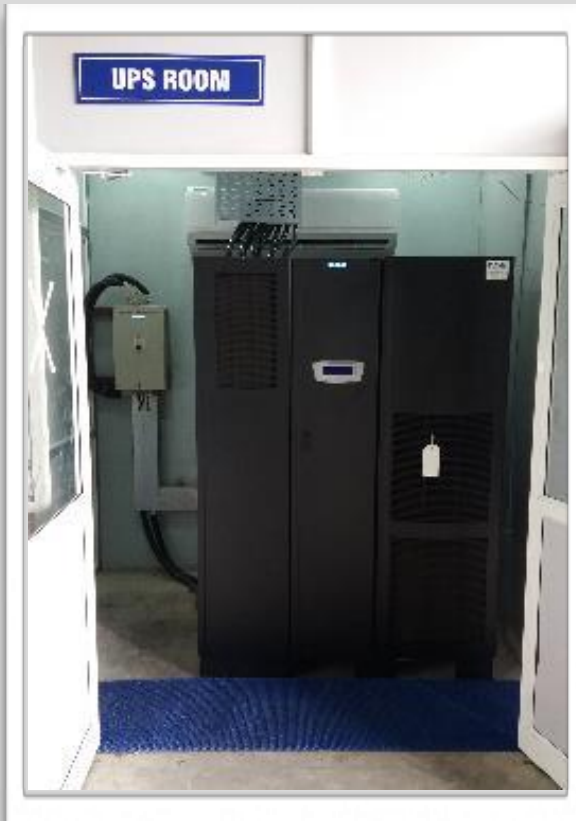
275KVA Power Backup for Die casting Machines
