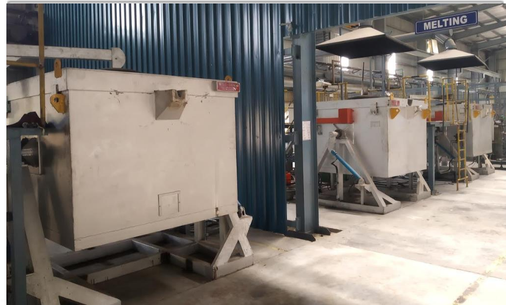
250Kg/hr Electrical fired Furnace – 3nos
