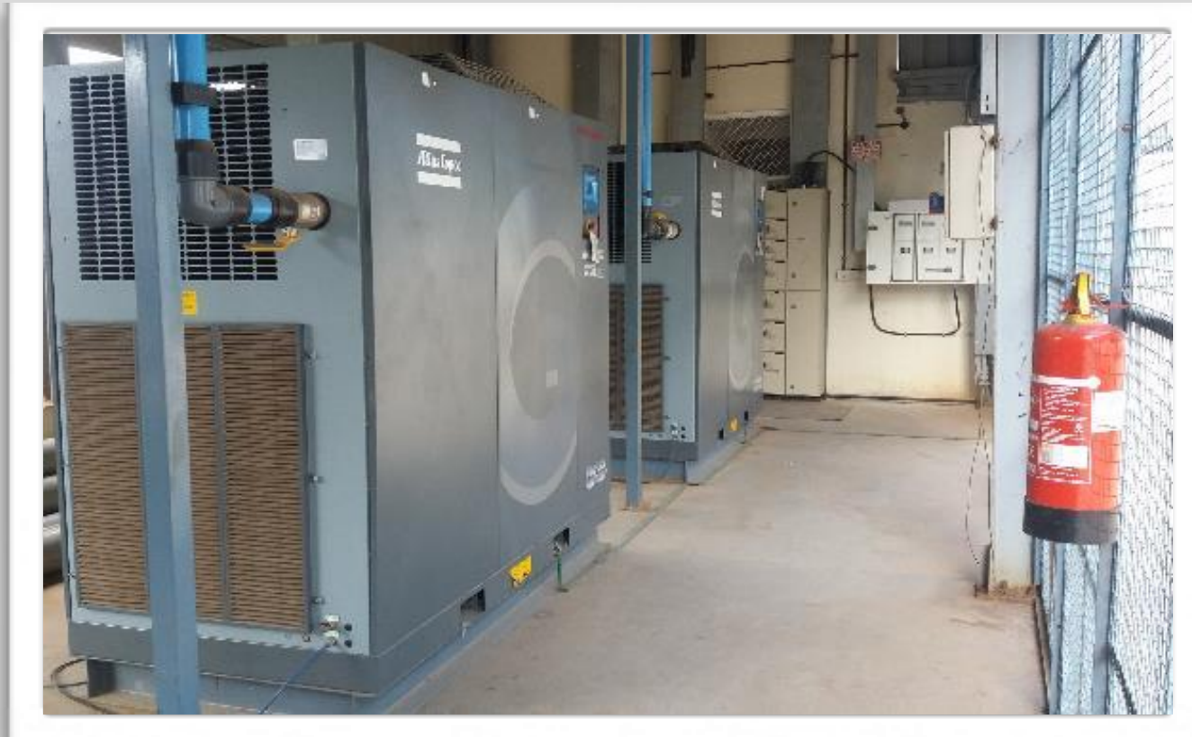
100HP Atlas Capco Compressor – 2nos
