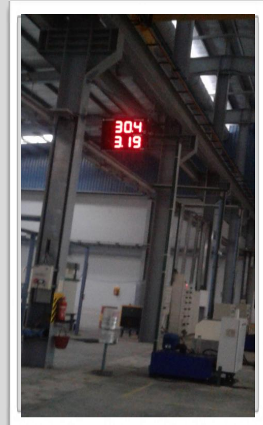
Temperature & Pressure Monitoring @ Shop floor
