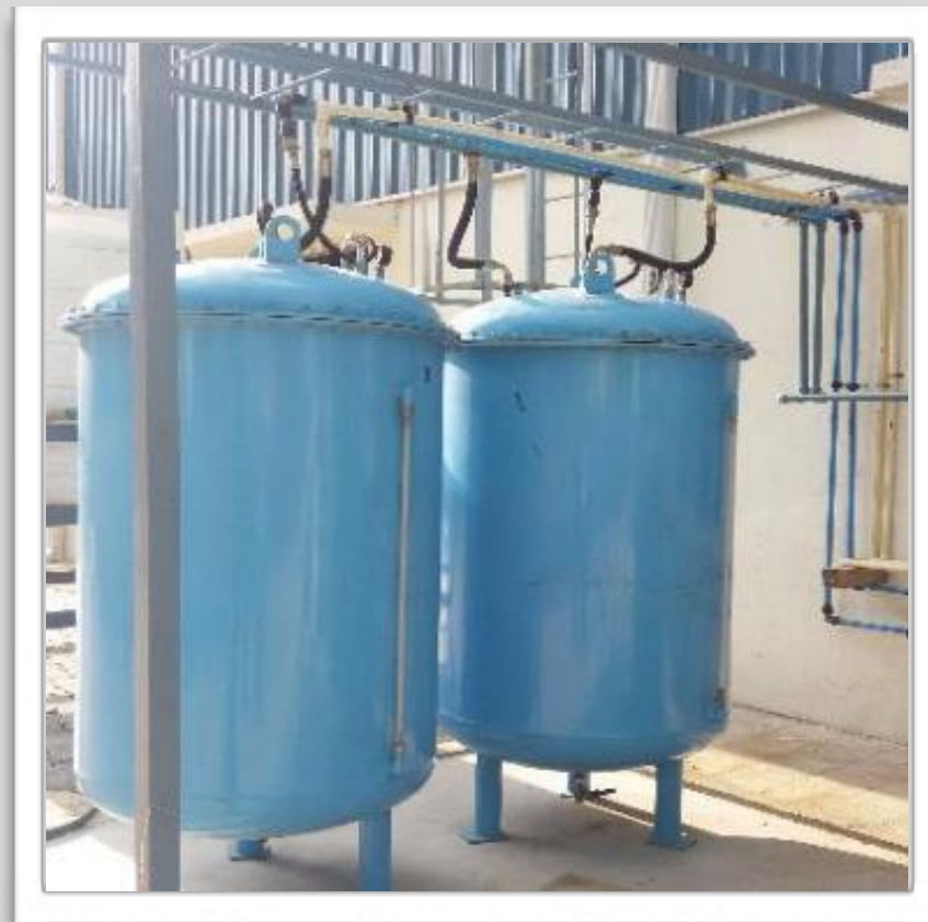
Die Coat Storage Tank
