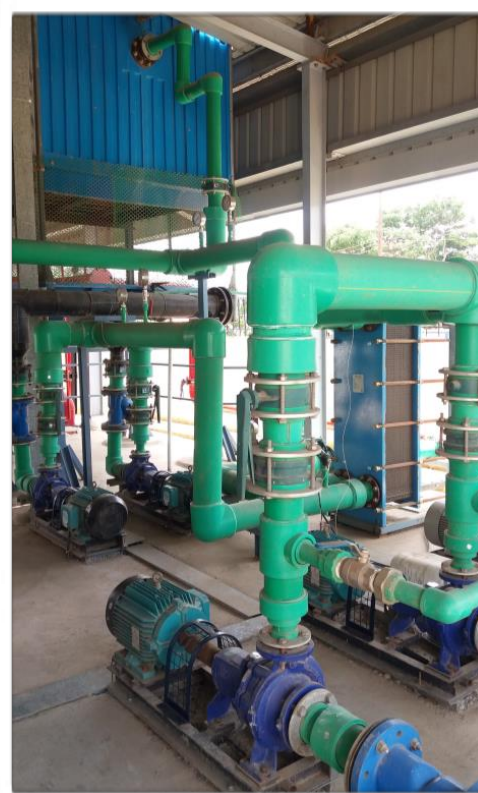
PHE Closed Loop Cooling System
