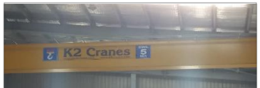
5T Crane -1no
